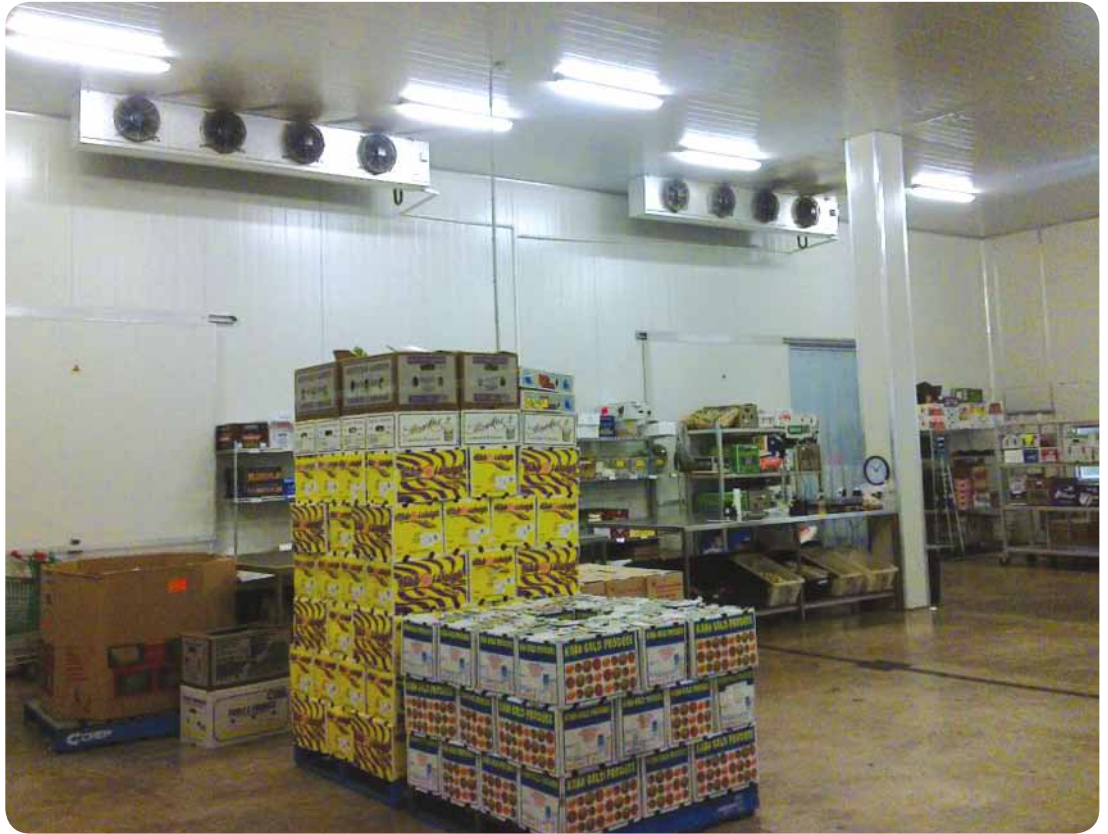
Two evaporators are utilised in the mango room.
