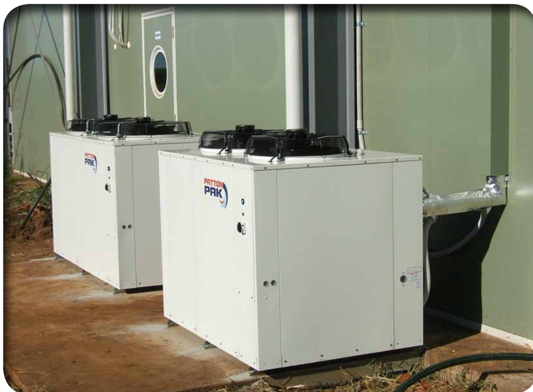
The cool room’s outdoor units.
